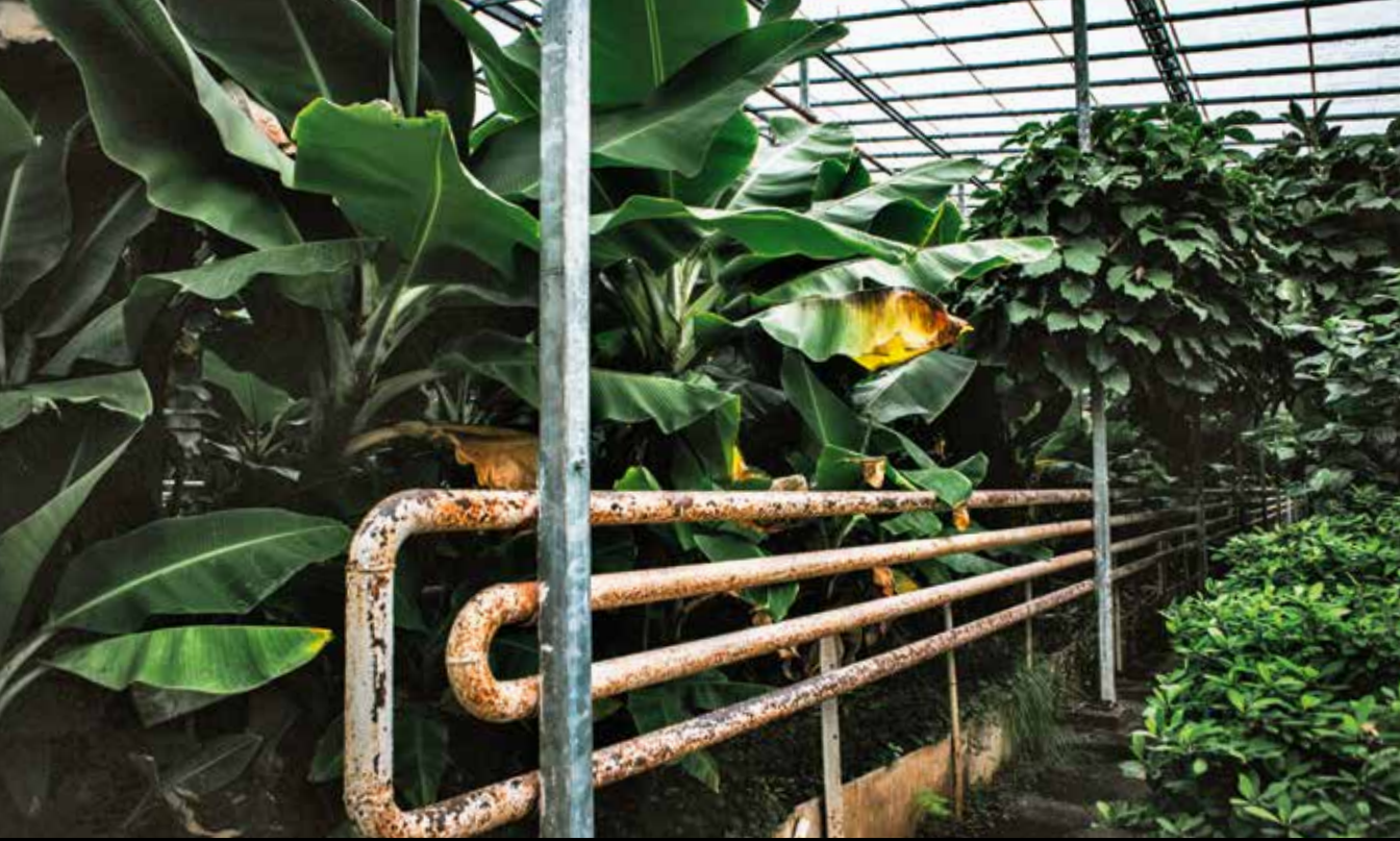
Geothermal energy used to heat a greenhouse.
