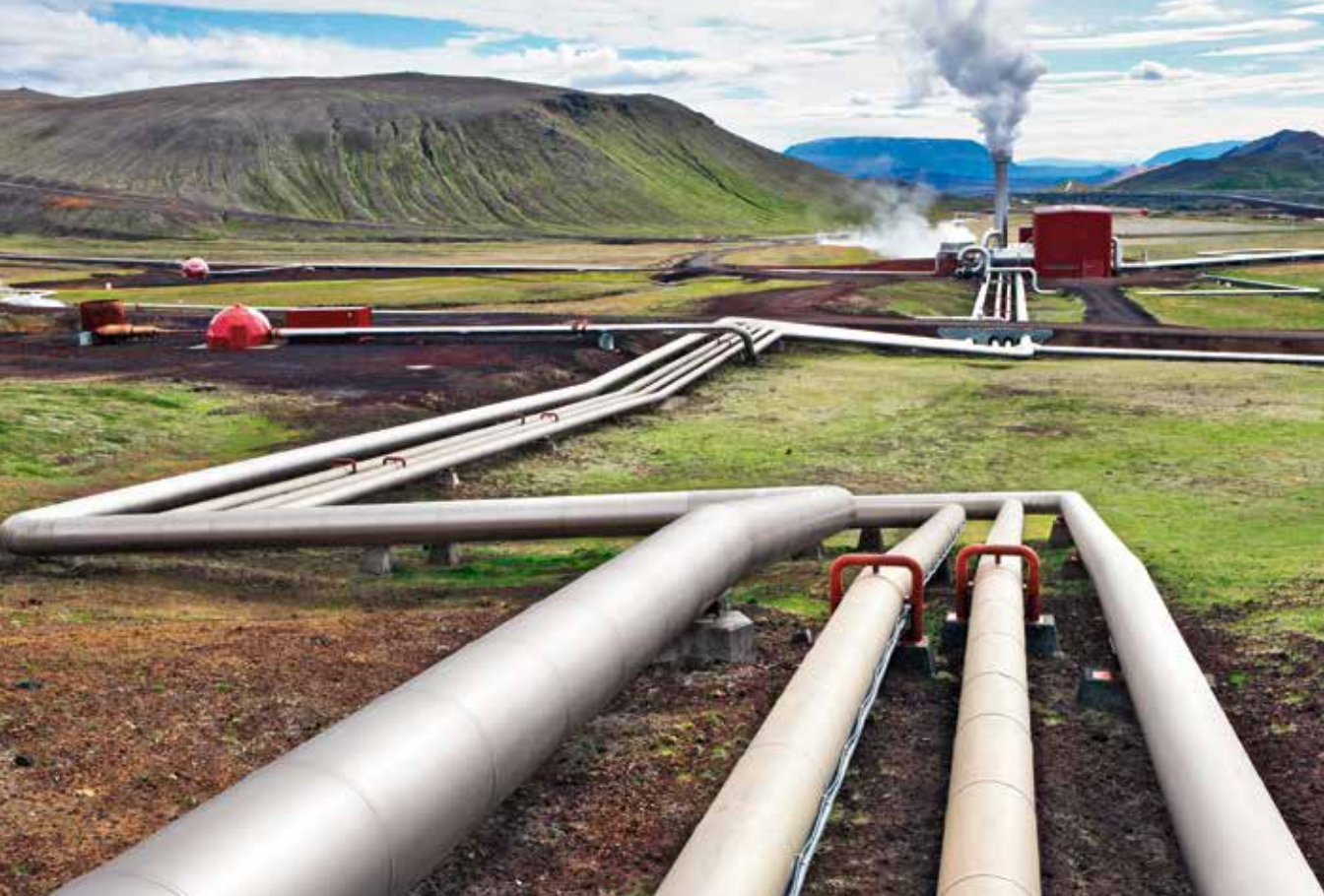
High-pressure steam being moved from boreholes to Krafla geothermal power plant in Iceland.
