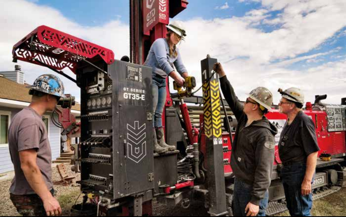
The U.S. gets into the act, here, drilling a hole for a geothermal heat pump installation in Hamilton, Colorado.
